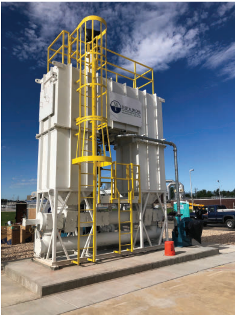
A regenerative thermal oxidizer is used to combust the low BTU tail gas produced by the gas conditioning system. Becky Luna/Carollo
