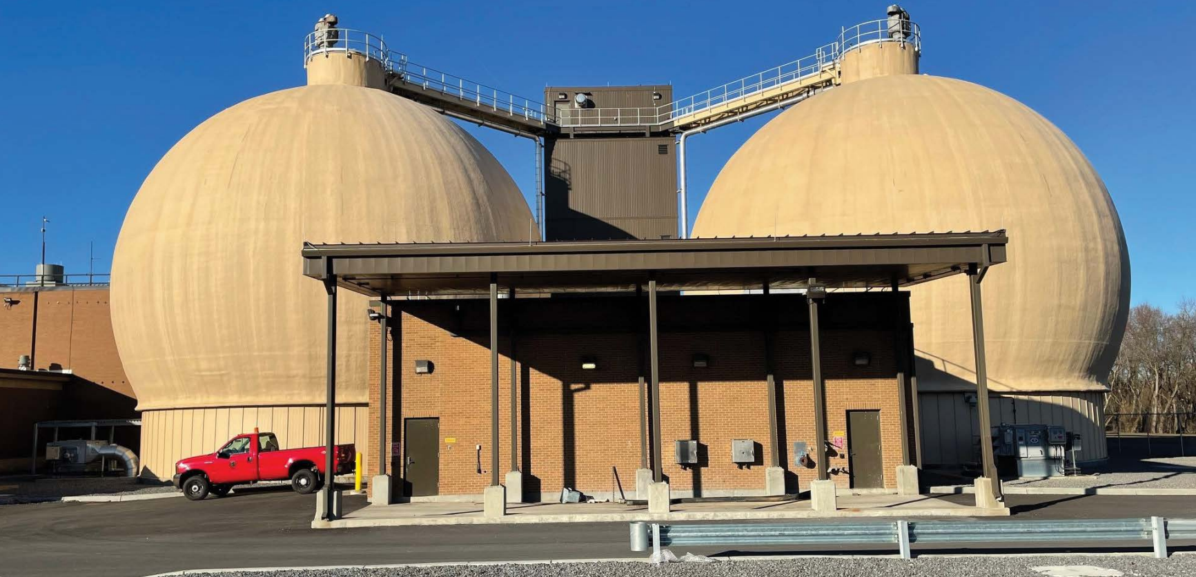
Figure 3. Anaerobic digesters were added to the Oneida WPCP to co-digest food waste. Credit: Oneida County Water Quality and Pollution Control
